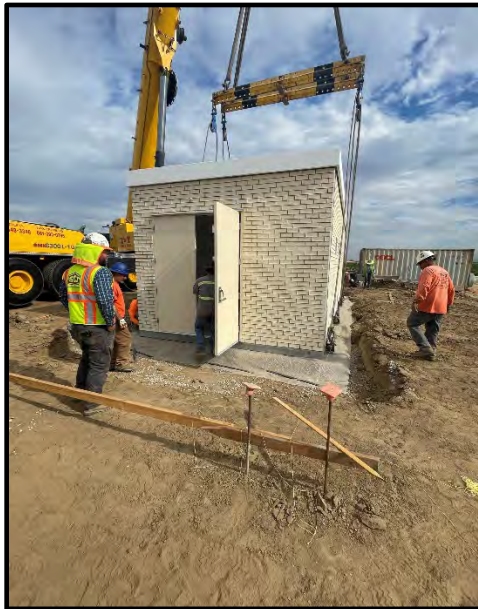
Photo 59: Pump House set.
