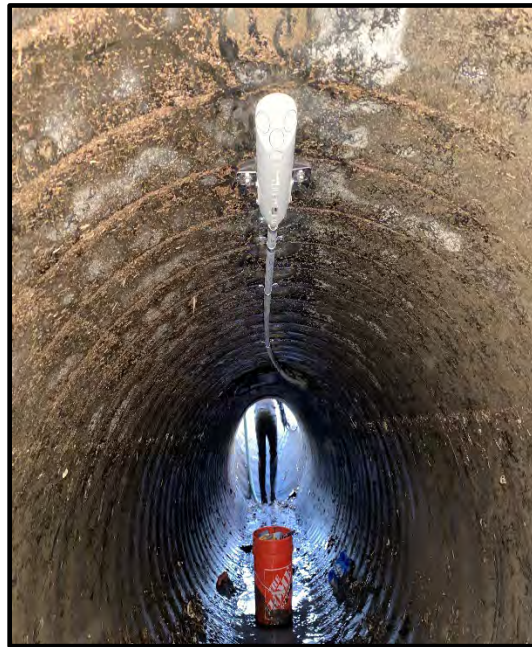
Photo 44: Typical pipe flow measuring set up.
