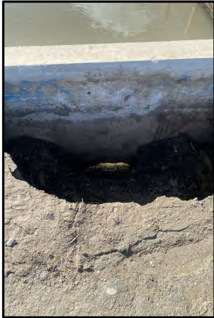
Photo 38: Close up of sinkhole, south headwall.
