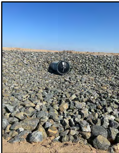
Photo 61: Discharge into Pond 2 with rip/rap.
