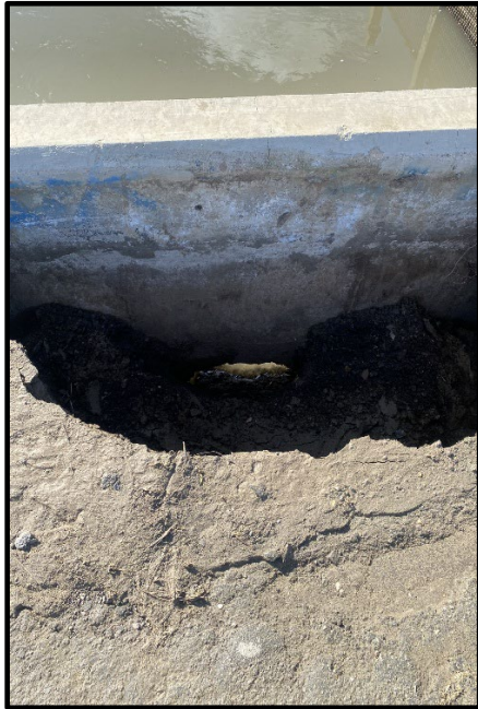
Photo 38: Close up of sinkhole, south headwall.
