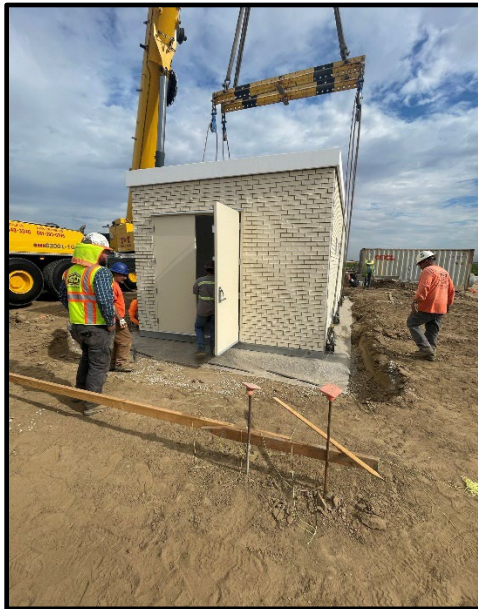
Photo 59: Pump House set.
