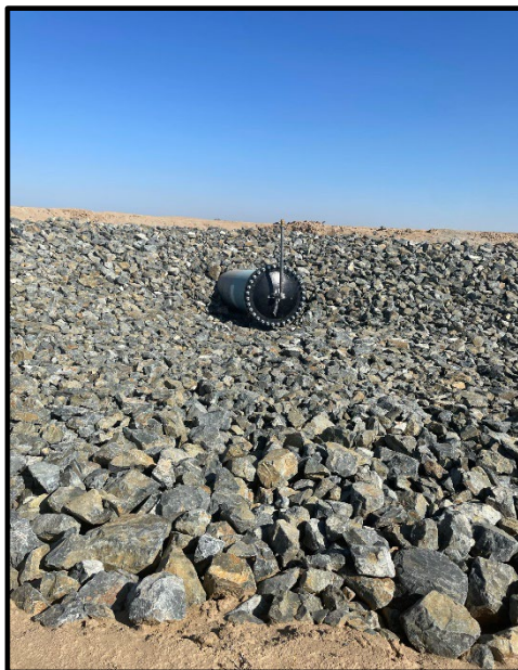
Photo 61: Discharge into Pond 2 with rip/rap.
