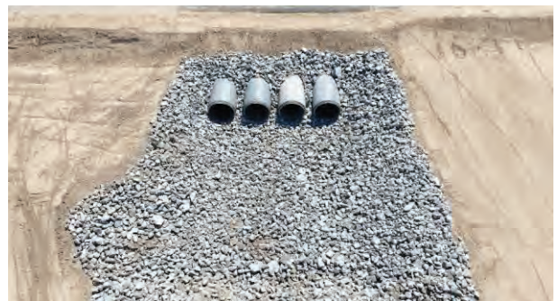
North Pioneer turnout outlet piping and rock slope protection.
