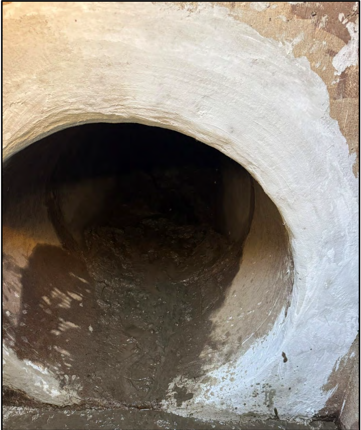
Showing the sealed crack around the 48-inch Hirshfield pipeline inside the manhole.
