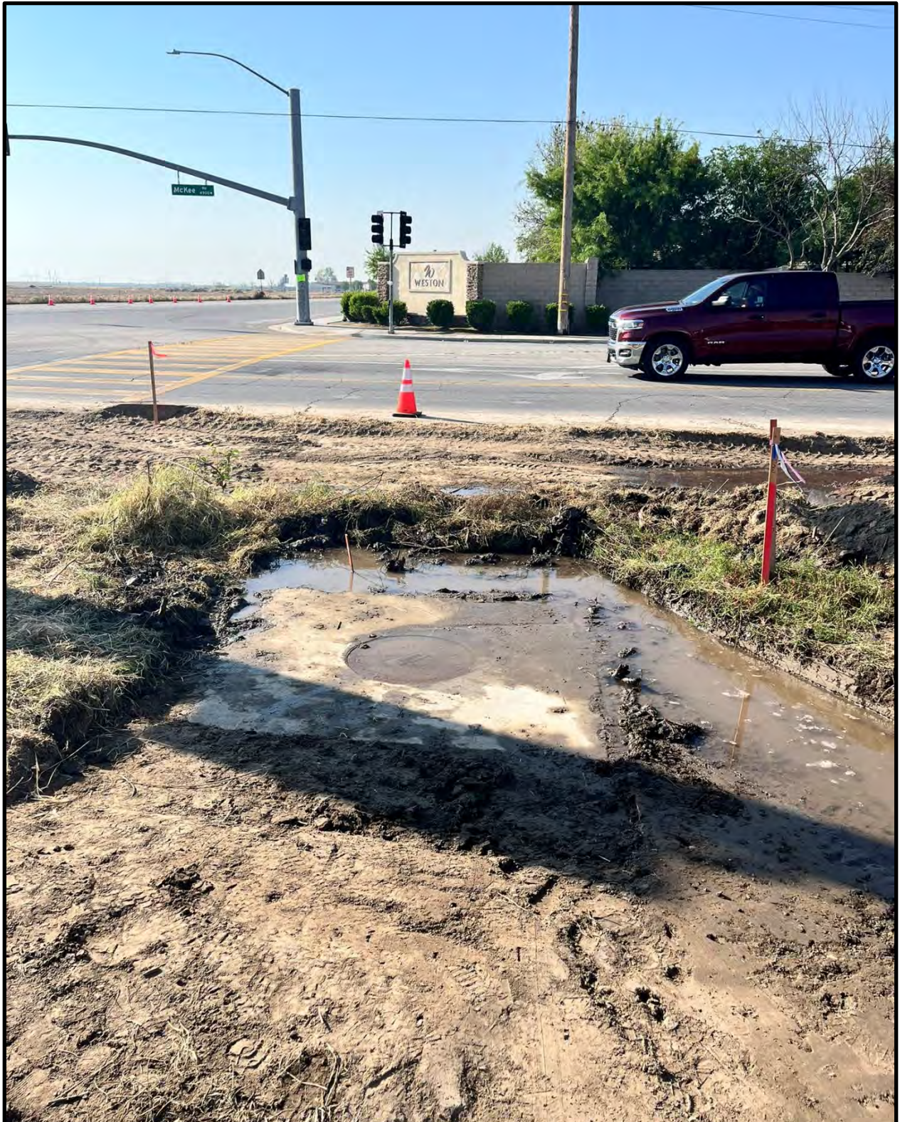
Looking south at the Hirshfield/Randall manhole leak.
