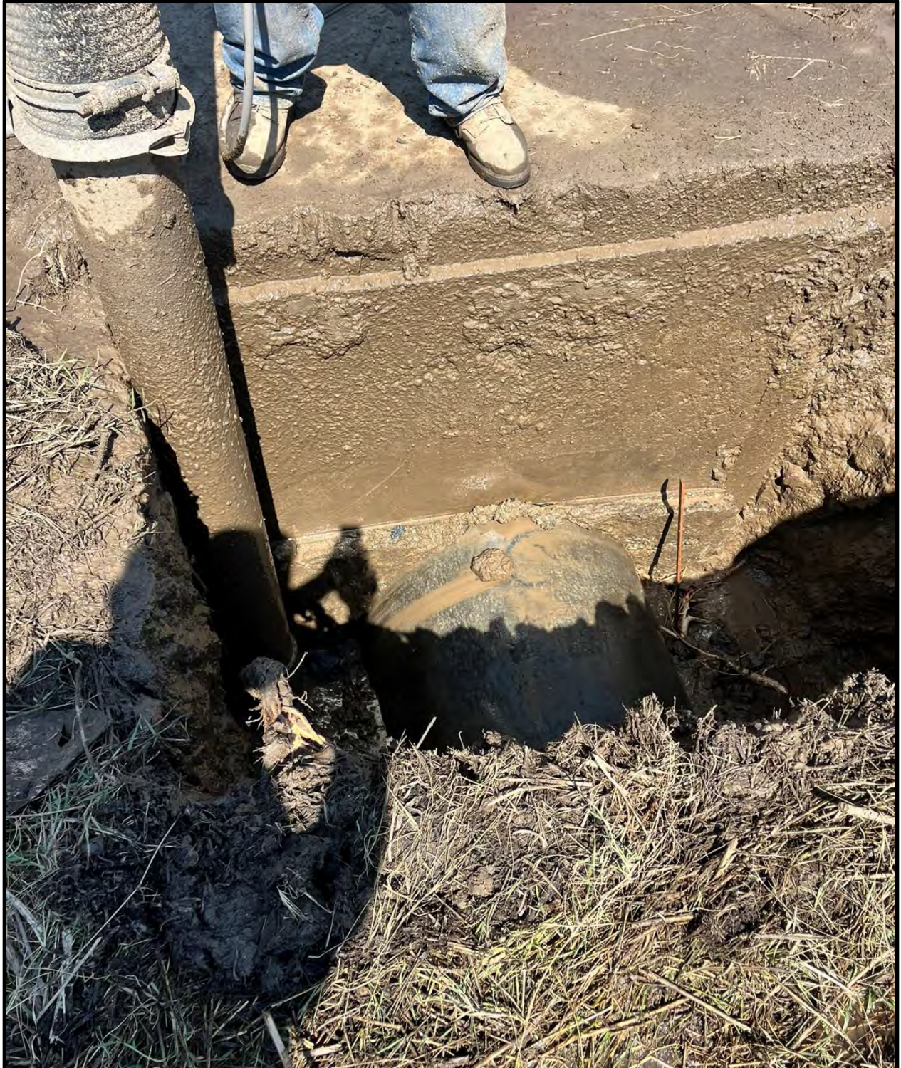
Looking north at hydrovac exposing leak at Hirshfield-Randall manhole. 36-in Randall pipeline shown.
