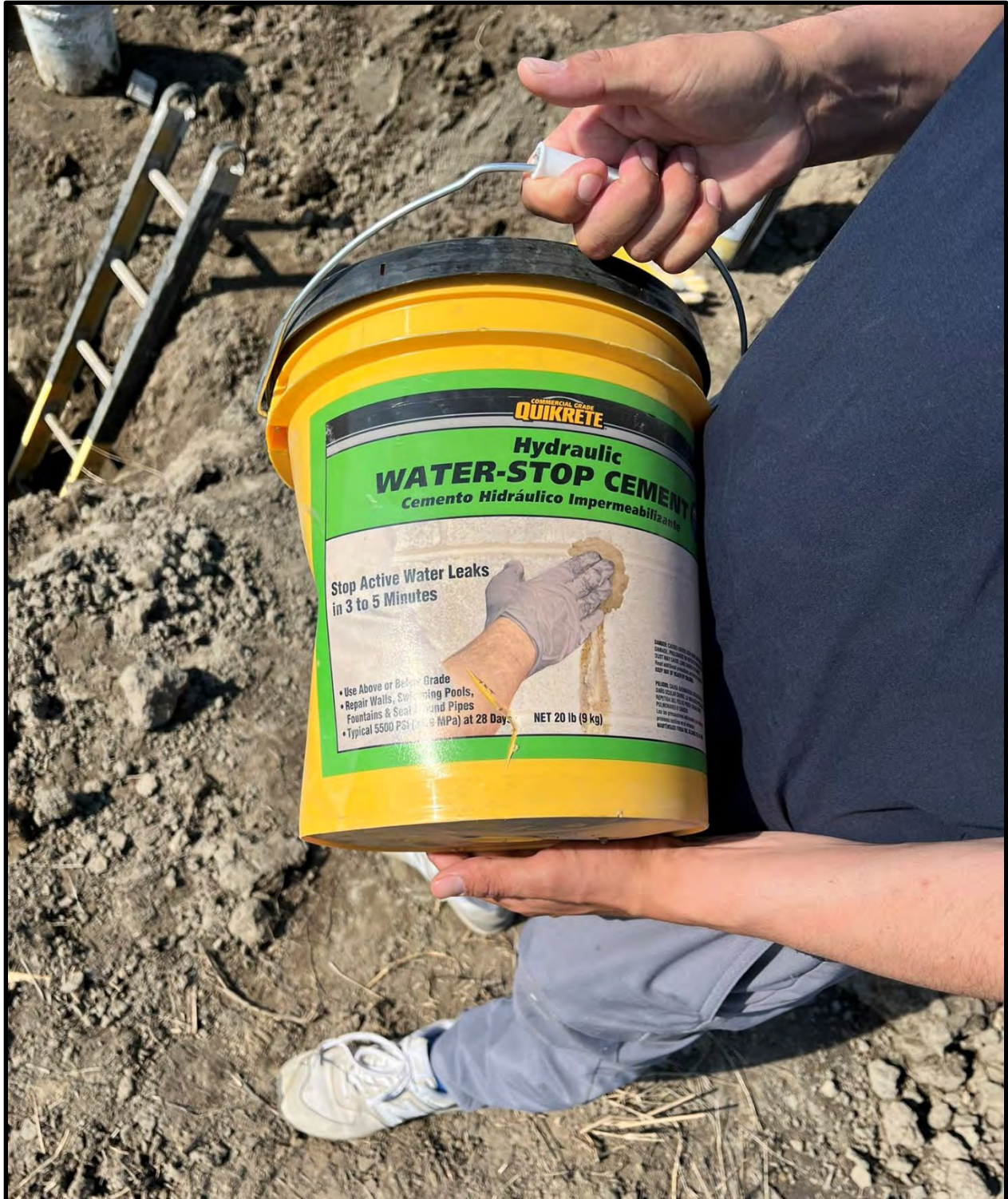
Hydraulic cement used to seal one joint that had water dripping during the repair.
