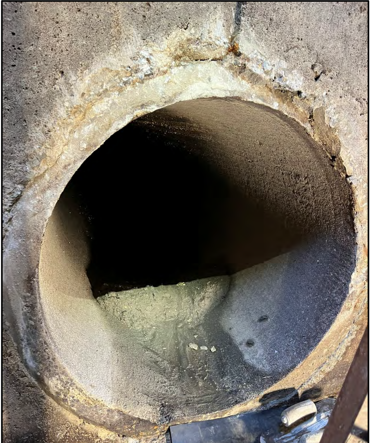
Showing cracks inside the manhole. Looking at the 48- in Hirshfield pipeline
