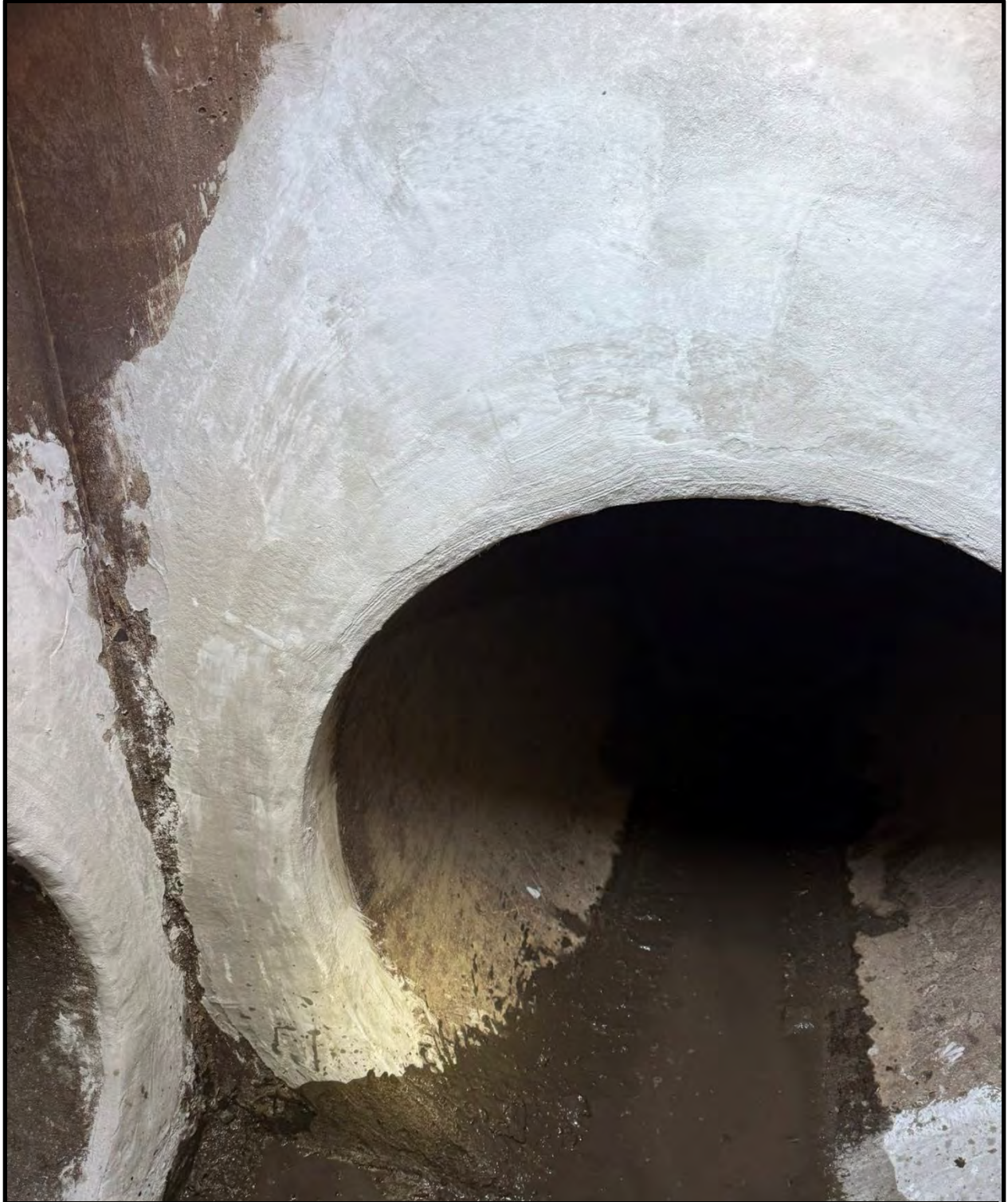
Showing the sealed crack of the 36-inch Randall pipeline inside the manhole.
