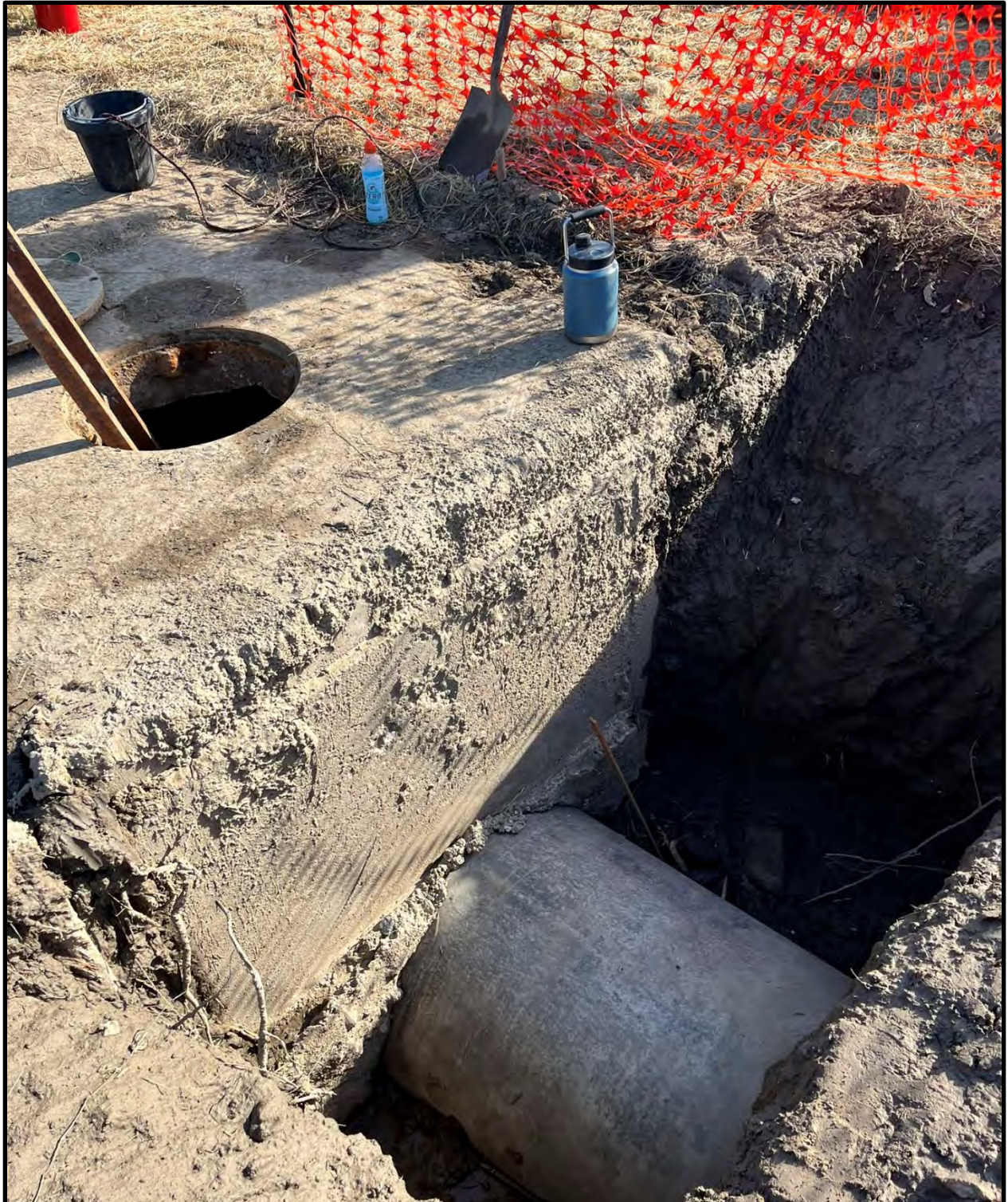
Showing the 36-in Randall pipeline exiting the south side of the manhole.
