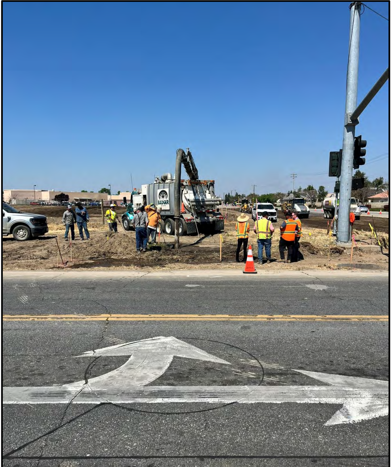
Looking north across McKee Road at hydrovac removing soil from the Hirshfield/Randall manhole.
