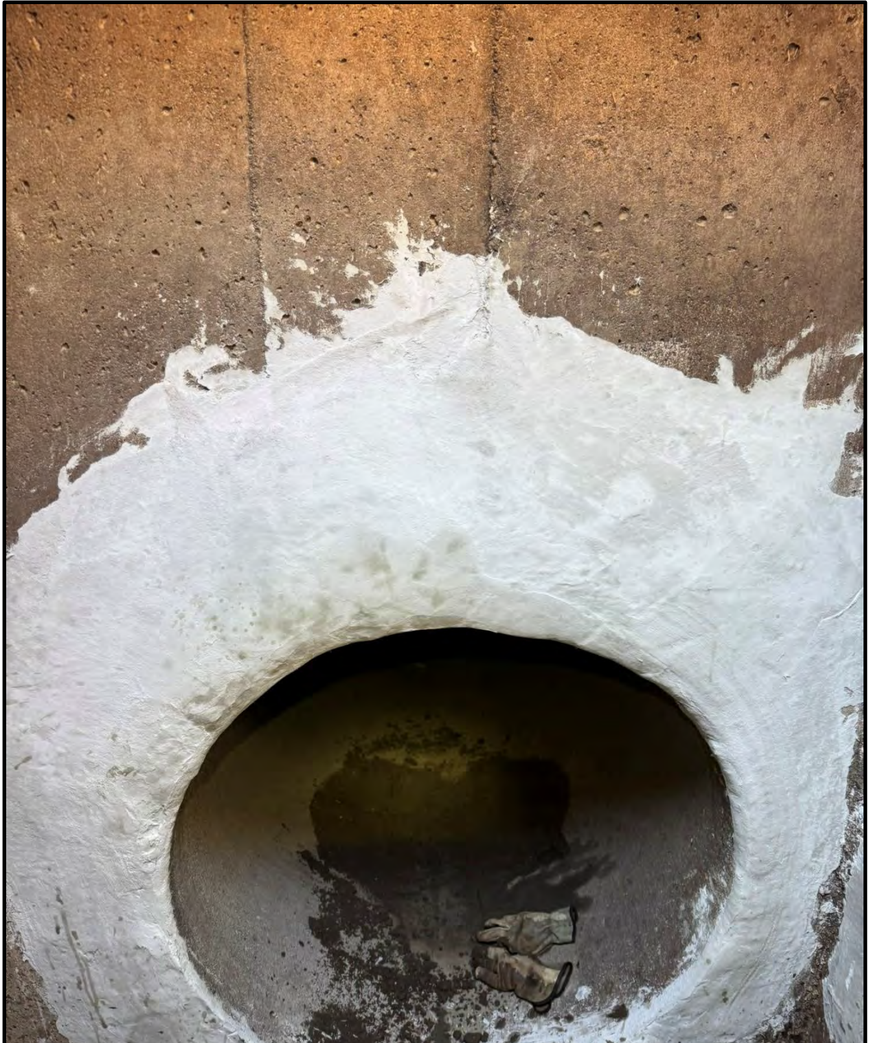
Showing the sealed cracks of the 36-inch Randall pipeline inside the manhole.
