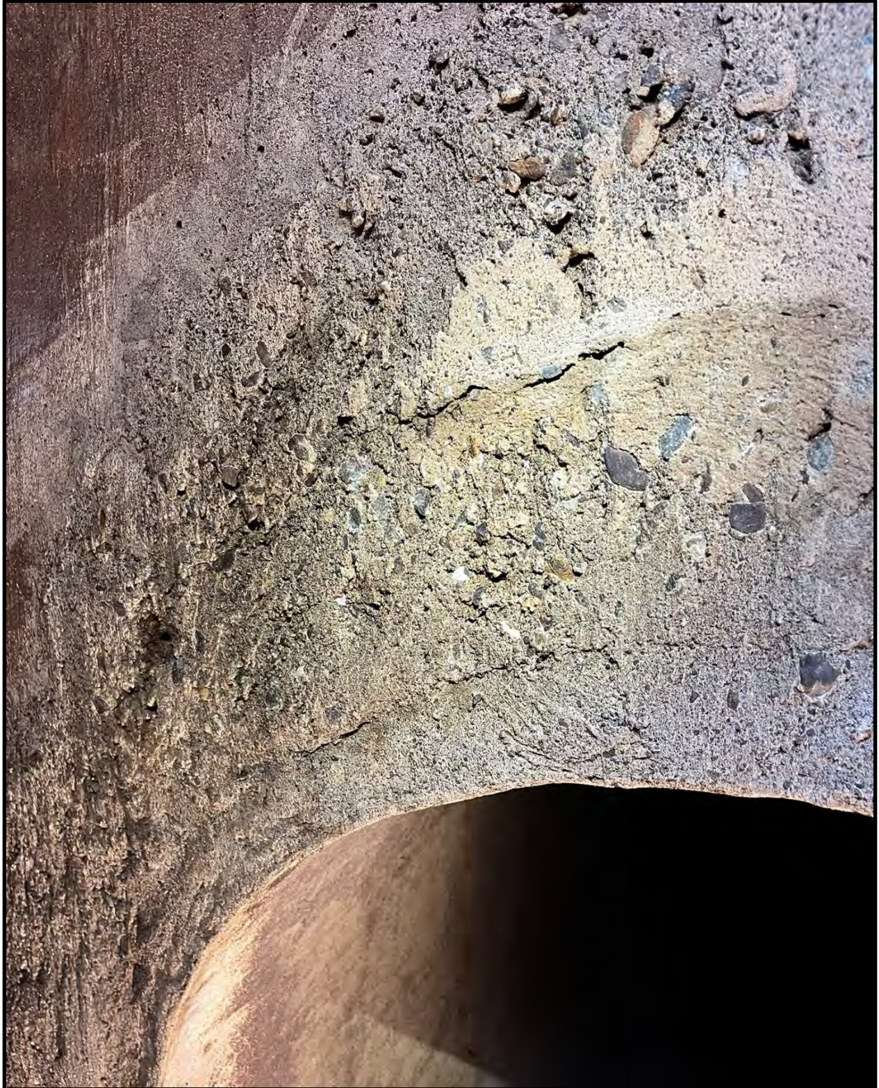
Showing cracks inside the manhole.
