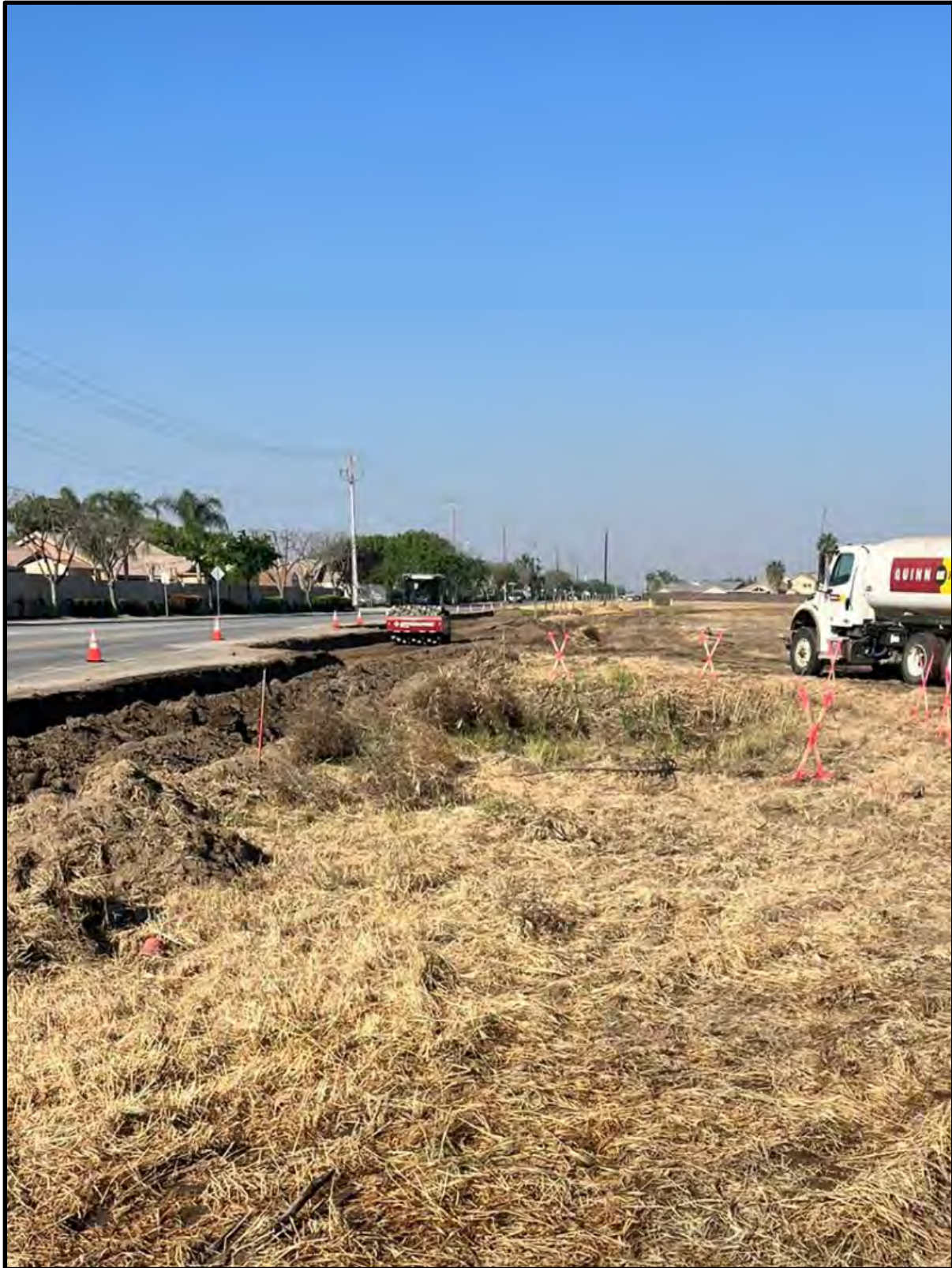
Looking west at the Hirshfield pipeline leak.
