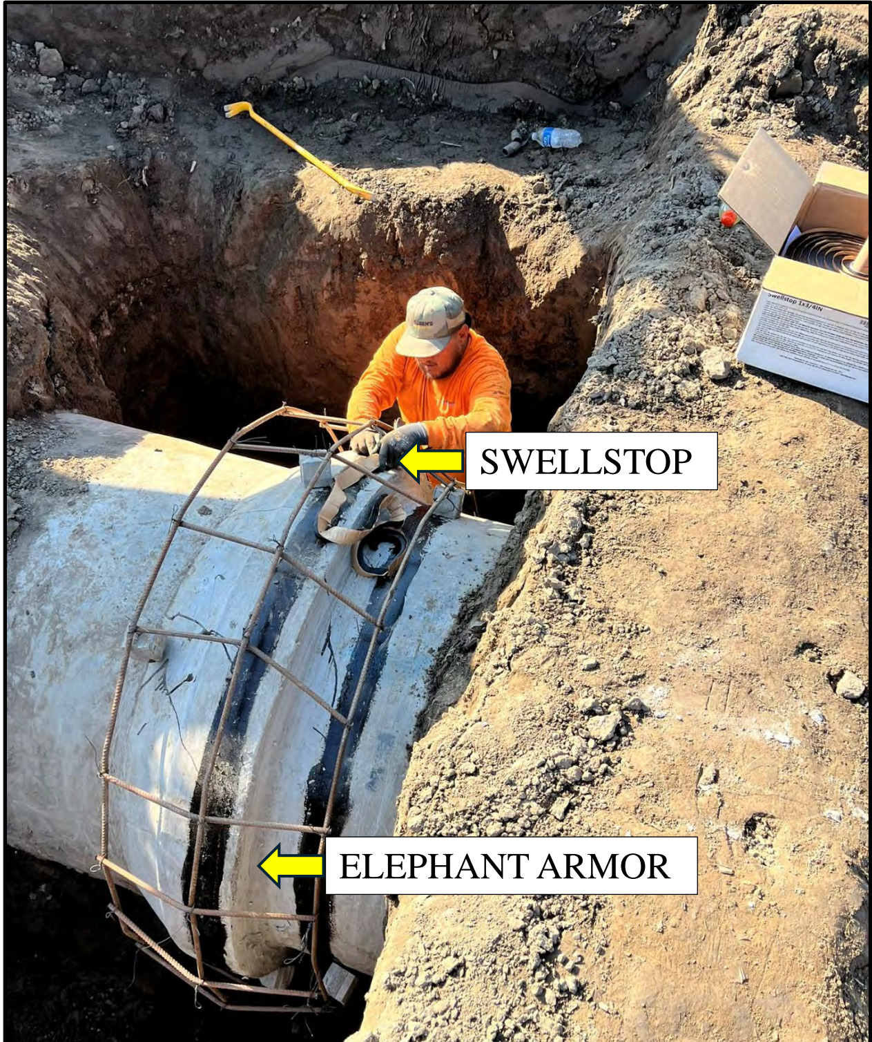
Showing the Swellstop installation process and the Elephant Armor joint sealant in the gaps.
